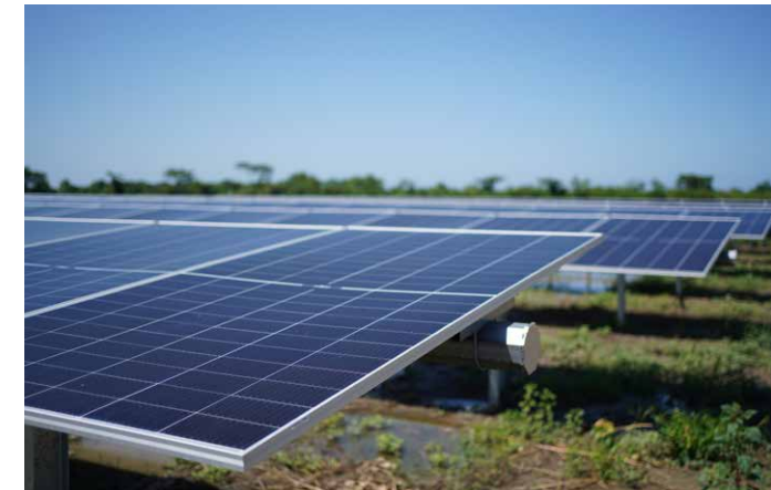
Solar photovoltaic power plant, Caimán Cienaguero (14MWp) - Colombia
